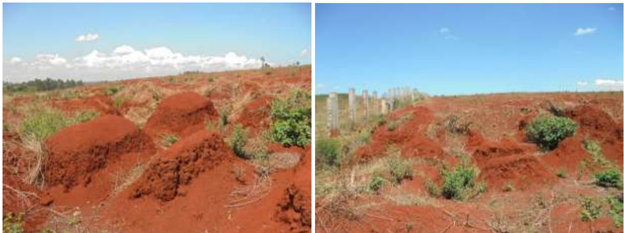
-View of collapsed foundations-
